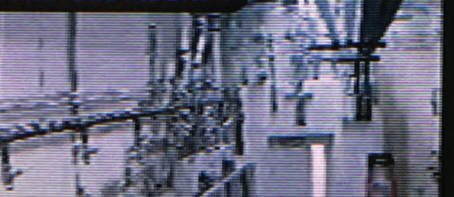
21 ISEB Gas Room 1
